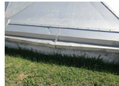
Primary Clarifier Dome
