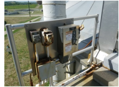
Electrical Box at Entrance to Primary Clarifier
