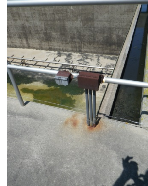
Electrical Junction Box at Aeration Basin #4A
