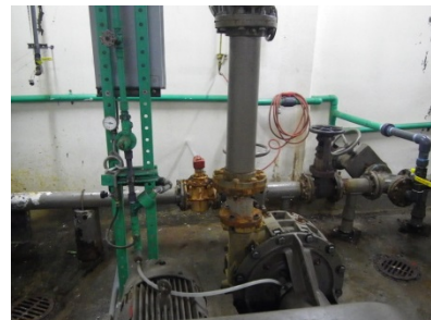
Grit Pump and Discharge Valve
