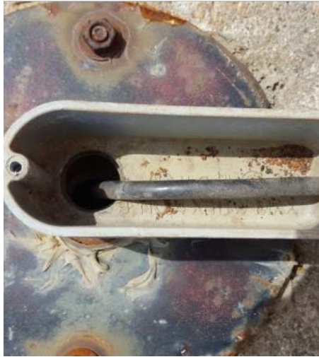
No Electrical Seal-Offs Between Wetwells and Control Panel
