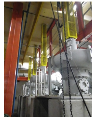
Trickling Filter Humus & In-Plant Waste Pumps #1, #2, & #3
