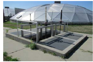
Slide Gates of Splitter Manhole #3
