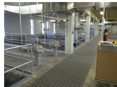
Effluent Filter Room
