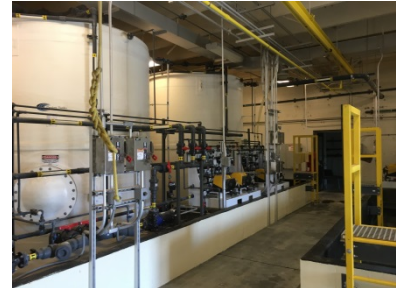
Sodium Hypochlorite Feed Pumps and Storage Tanks
