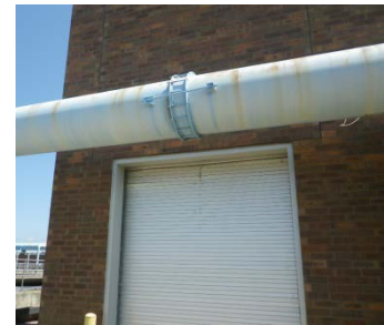
Aeration Header Piping
