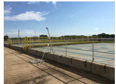
Chlorine Contact Basins
