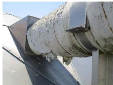
Odor Control Ductwork
