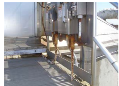
Electrical Conduits at Platform
