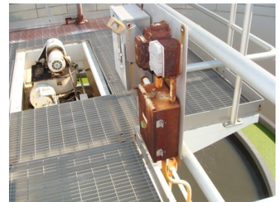
Electrical Box on Walkway of First Stage Intermediate Clarifier #2
