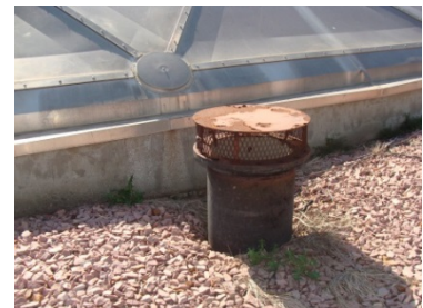
First Stage Trickling Filter #1 Vent
