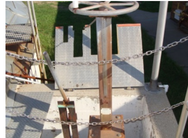
Primary Clarifier #1 Telescoping Valve Operator
