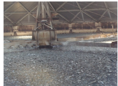
First Stage Trickling Filter #1 Rotary Distributor
