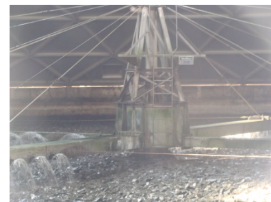
Second Stage Trickling Filter #1 Rotary Distributor
