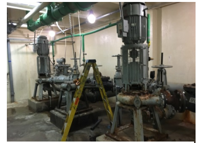
In-Plant Waste Pumps #1, #2, & #3
