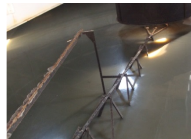
Primary Clarifier #4 Rake Arm
