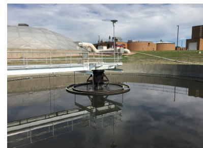
Second Stage Intermediate Clarifier #2
