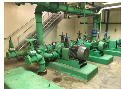
Non-Potable Water Pumps #2, #3, & #4
