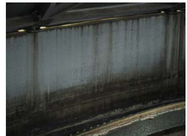
Interior of Clarifiers
