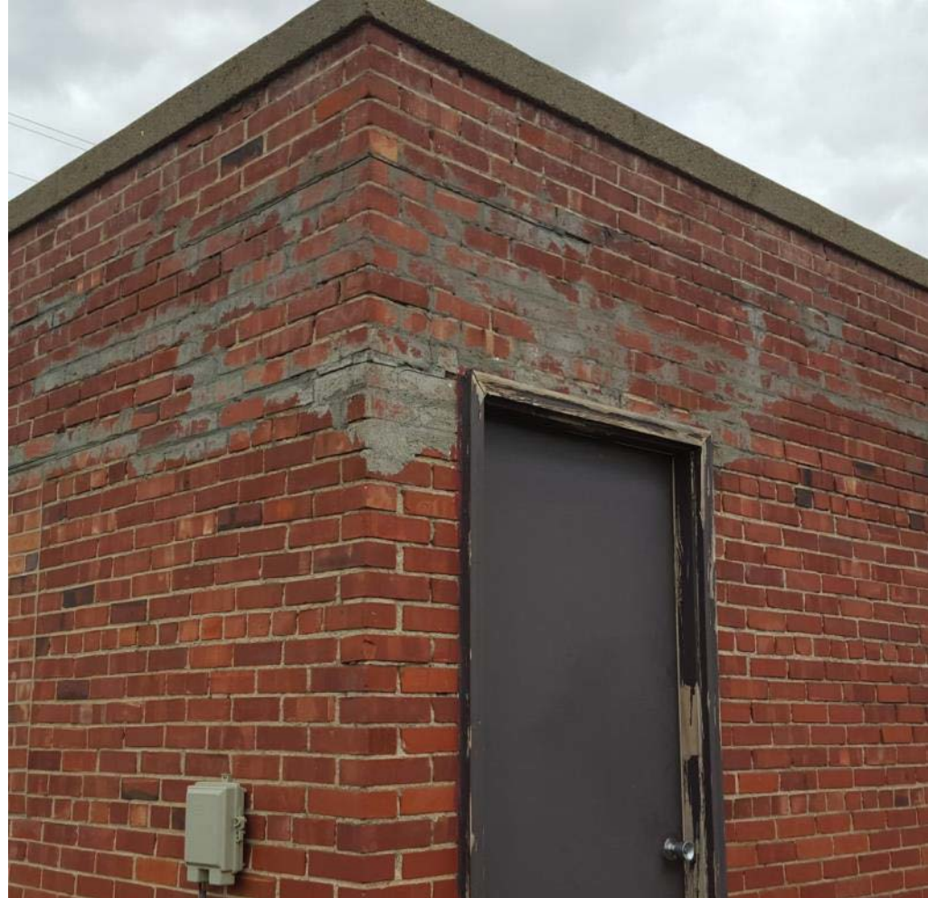
Structural Condition Poor – Needs a complete Rebuilt
