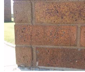
Crack in Exterior Wall
