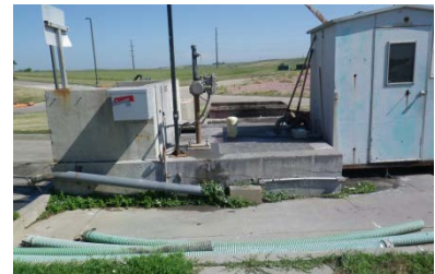
Septage Dumping Station
