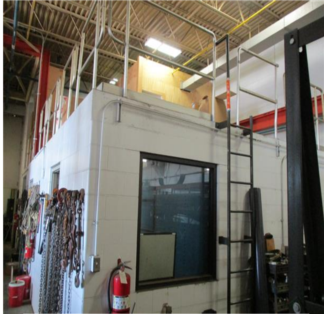
Mezzanine – Missing Ladder Rail and Toe Plate
