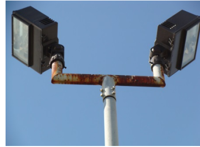
Light Fixture Support at Manhole #9
