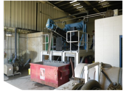
Grit Cyclones and Grit Washer at the EQ Basins
