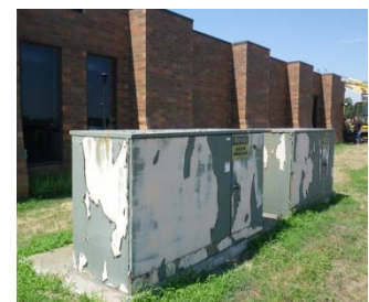
Electrical Transformers at the RAS Building
