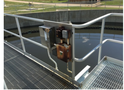
Electrical Box on Walkway of Second Stage Clarifier #1
