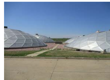
First Stage Trickling Filter Domes
