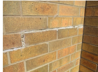
Water Damage to Brick Veneer
