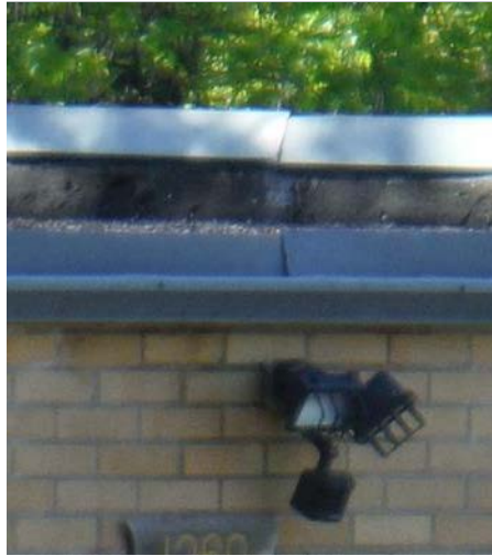
Deterioration of Roofing Material
