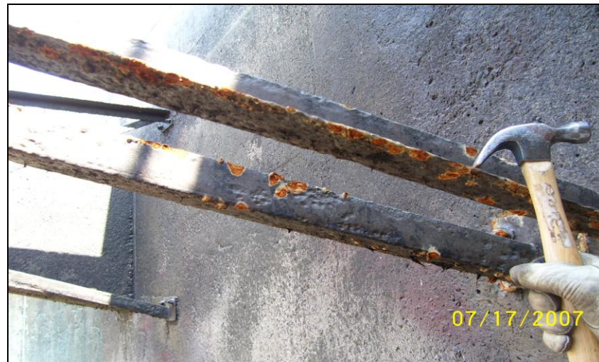
Figure 20 Final Clarifier #1 Scum Box Support Arms
