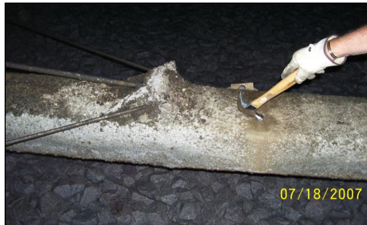
Figure 15 Trickling Filter Arm Corrosion
