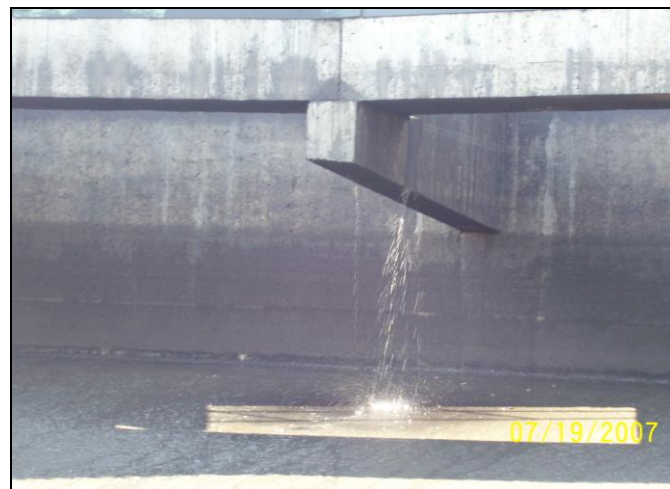
Figure 18 First Stage Intermediate Clarifier #1 Effluent Trough
