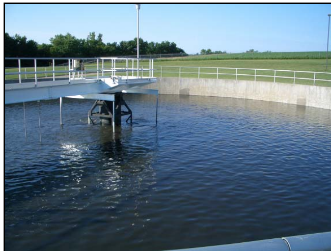
Figure 31 Second Stage Intermediate Clarifiers at 27.125 mgd
