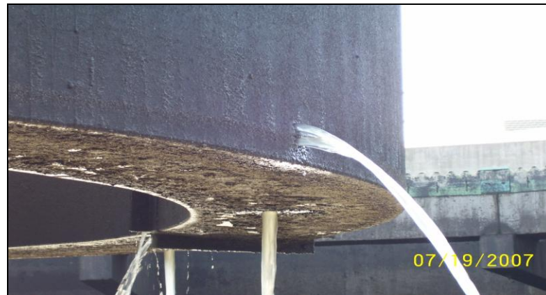
Figure 17 First Stage Intermediate Clarifier #1 Influent Well
