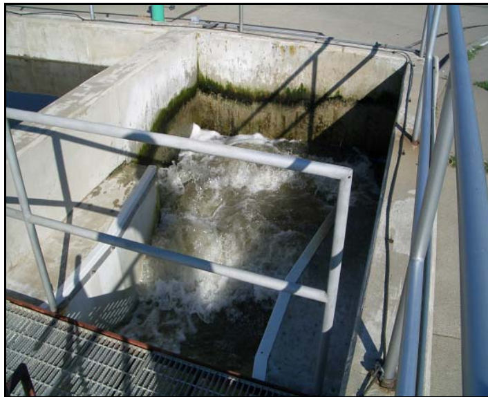
Figure 32 Effluent Flume at 27.125 mgd
