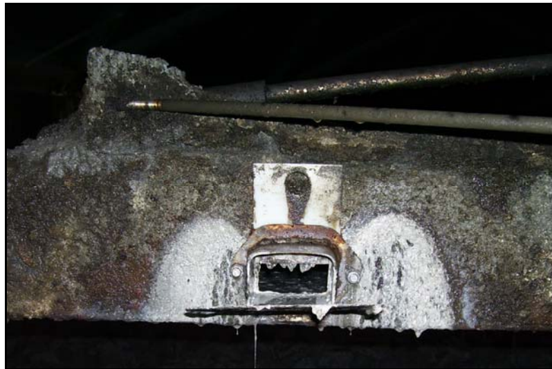
Figure 17 First Stage Trickling Filter Distributor Corrosion
