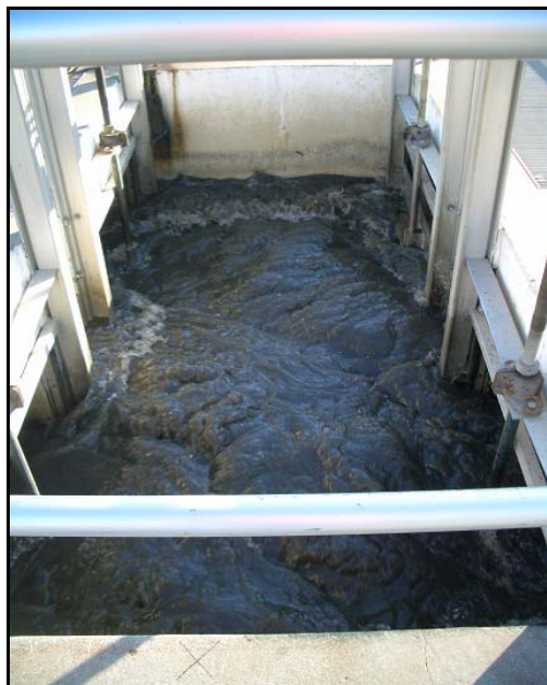
Figure 15 Typical Wave-action in Splitter Manhole No. 3
